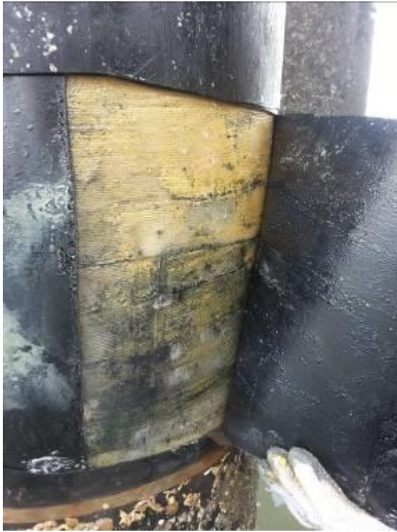
Photo 25: Ingress of Mud into STACwrap
