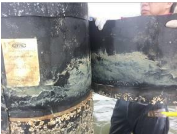
Photo 23: Ingress of Mud into Overlap
