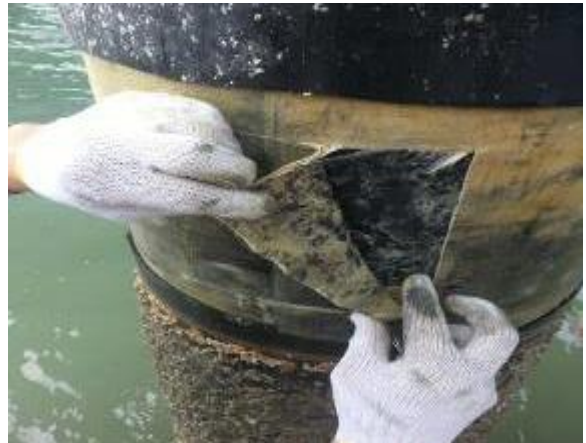
Photo 30: Cut off Section of STACwrap
