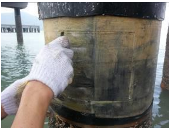
Photo 29: Cut off Section of STACwrap
