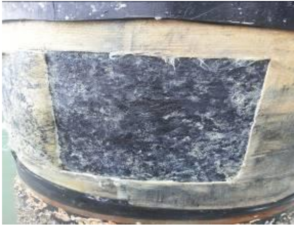
Photo 31: Condition of Steel Pile Surface
