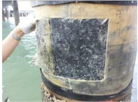
Photo 32: Condition of Steel Pile Surface
