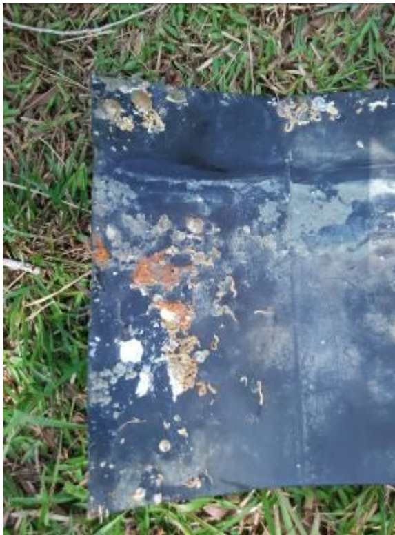
Photo 53: Sample of HDPE Jacket
